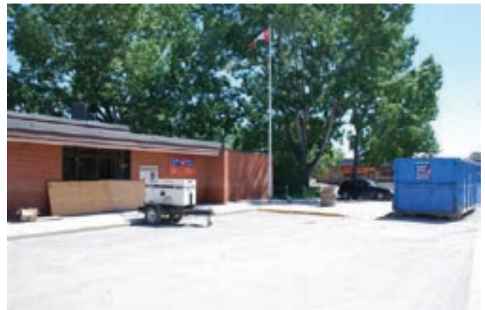
Figure 9 - flood damage, main post office.
